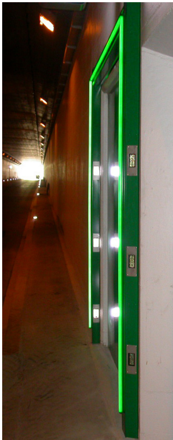
Example for integrated system consisting of LED Tube and Power LED Flasher - used in road tunnels
